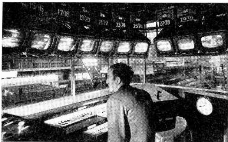
FIFTEEN closed-circuit television channels in the new rolling mill of the Steel Company of Wales at Port Talbot provide a composite view of about 700ft of railway track. This installation by Marconi's is for the remote observation of the conveyance of red-hot steel ingots from the soaking pits to the rolling mill.
